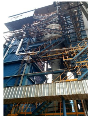
Gambar 2. Boiler PT. PHO
