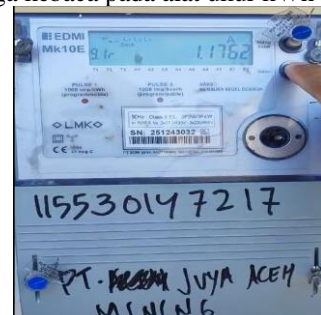
Gambar 3. kWh Meter PT.Juya Mining Aceh
