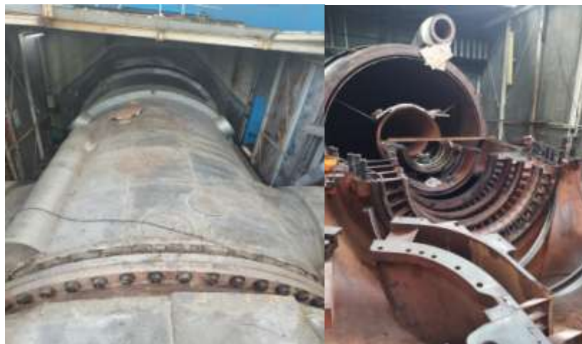
Gambar 2. Poros Turbine Uap dan Cover Bantalan Aksial (Thrust Bearing)
