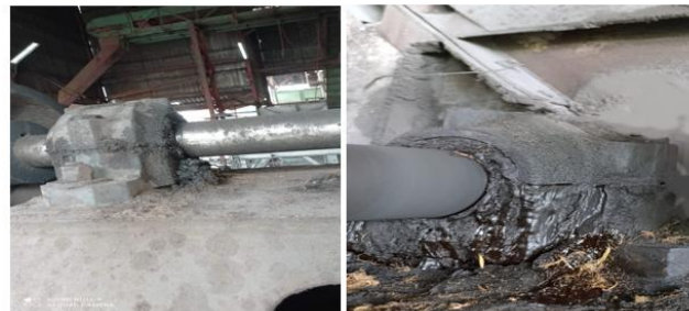
Gambar 8. Kondisi Pelumasan Grease Roller Bearing
