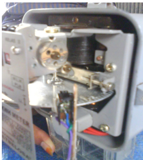
Fig 6. Modified KWH Meter
